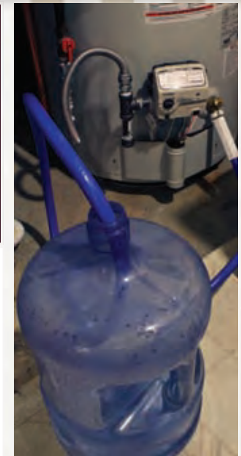
Know where your utilities are located and whether you have access to them or not. Access to your water heater — and a little knowledge — means you have a significant cache of potable survival water.
