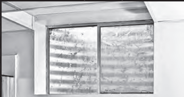
Interior window: This basement window is vulnerable to entry through the window well outside.
